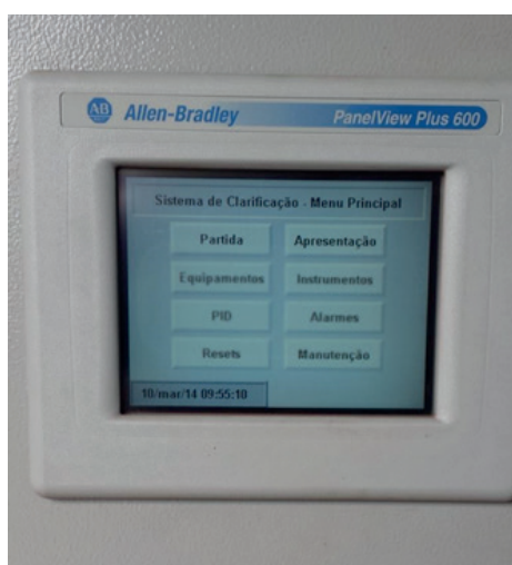
Figura 13– Monitor do PLC
